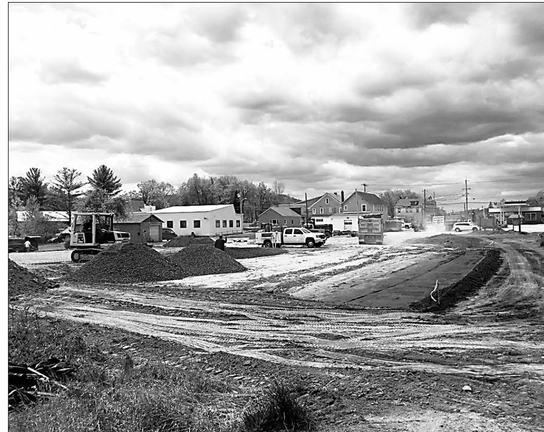
The Center for Discovery has begun paving the new basketball courts, located adjacent to the Rail Trail.
